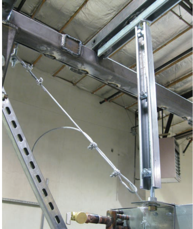
FIGURE 8 - UNISTRUT USED TO STRENGTHEN THE ROD
