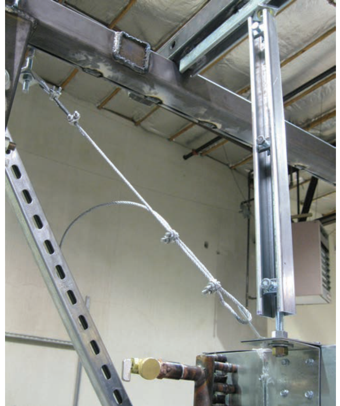
FIGURE 6 - UNISTRUT USED TO STRENGTHEN THE ROD
